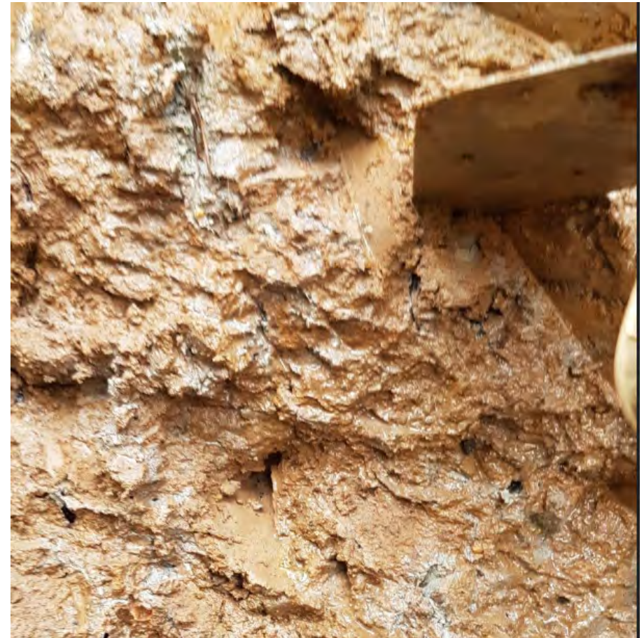
Photo 02: Possible 80 shallowing to 75 degree slip surface in-situ (non-annotated)
